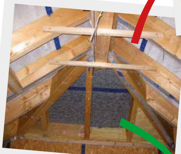
One roof, the same conditions, different results: pore-free SOLITEX MENTO membrane on the hip roof, microporous membrane on the main roof surfaces to the left and right.
